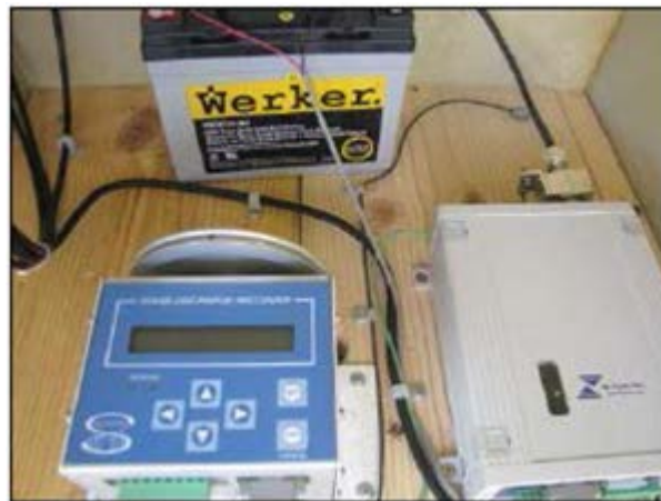
Flume equipment box with flume flow discharge readout. Radio or satellite signals are relayed by antennas from the flume data recorders and received by remote computer in Santa Fe every 15 minutes. Office of the State Engineer/Interstate Stream Commission uses the flow data to assist in administering water rights and managing water throughout the State
