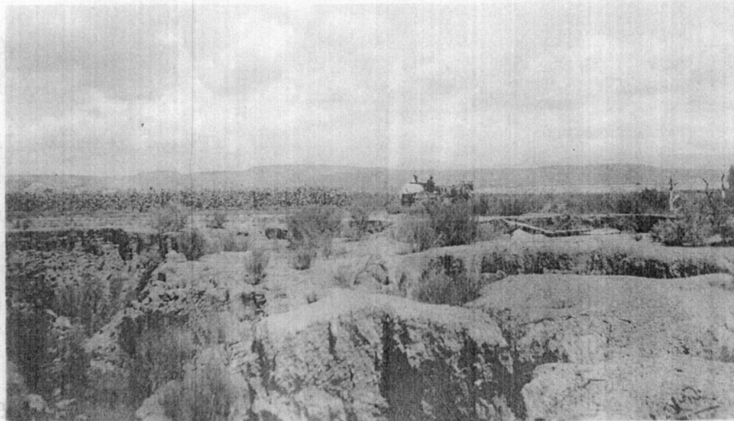
No. 16. Erosion caused by waste ditch on lands of the Pueblo of Jemez.
