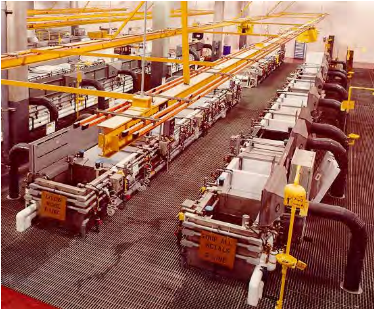
Corpus Christi Army Depot, Corpus Christi, Texas Advanced Metal Finishing Processes and Facility (original date: 01/26/1998; revision date: 04/14/2003)
