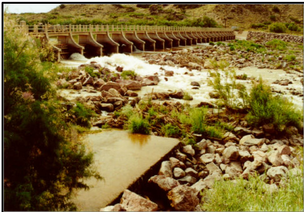
Plate A.24. View of San Acacia Diversion Dam (RM 116.2) that forms the boundary between geomorphic Subreaches 5 and 6. Note the riprap emplaced to counter the effects of channel degradation downstream of the structure.
