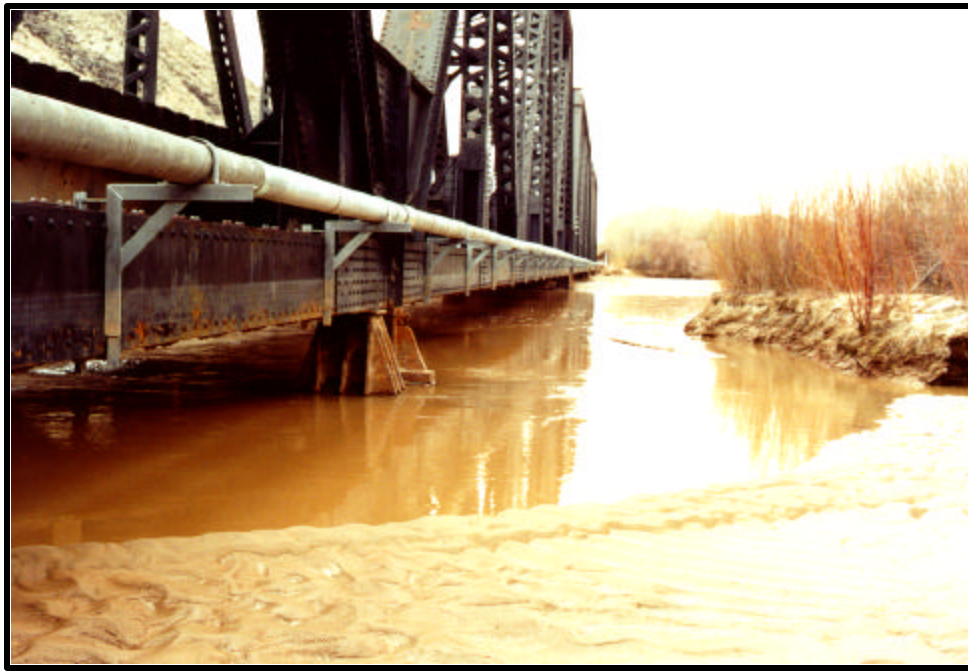
Plate A.35. View of the downstream face of the San Marcial Railroad Bridge showing the effects of aggradation.
