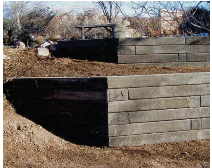
Figure 5-1: Retaining walls can reduce soil erosion and create additional spaces for plants and recreation areas.
